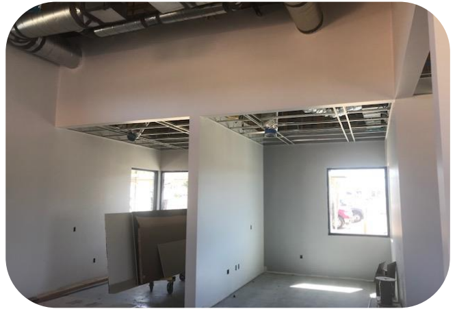
T-Bar Ceiling Grid
