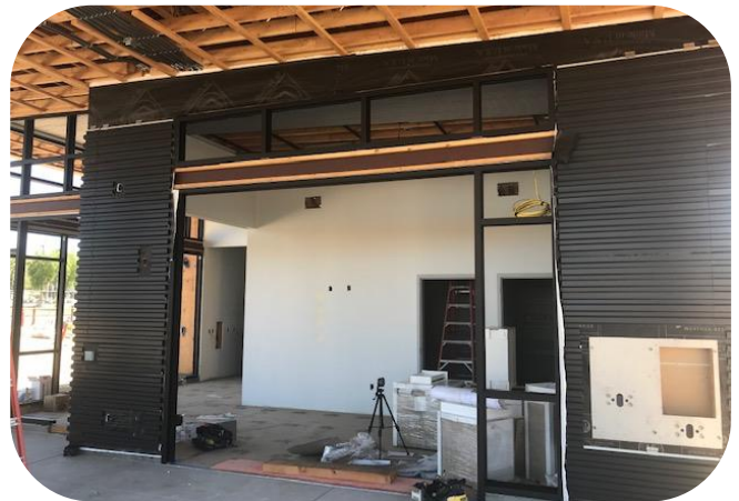
Sliding doors pending.
