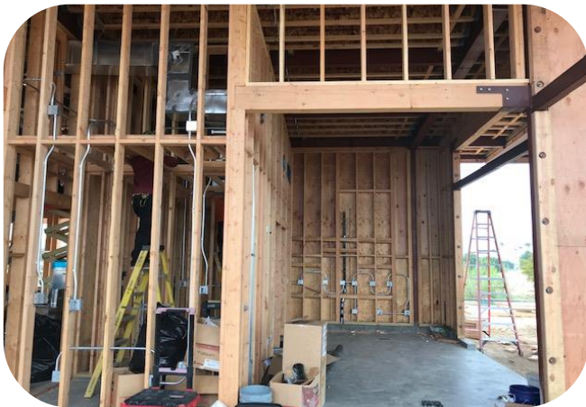
HVAC ductwork, electrical rough in
