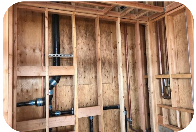
Plumbing waste/vent/ domestic water
